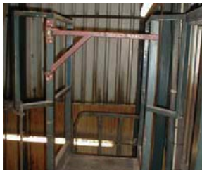
Fixed ladder safety bar
