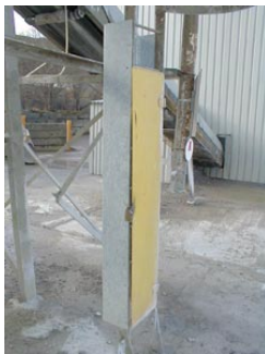
Preventing unauthorised ladder access
