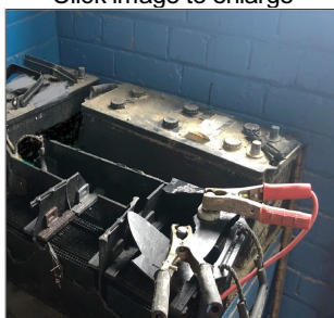
Photograph showing the damage to the battery casing after the explosion. Also shown is an intact battery with its six cell caps fitted.
