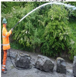
Picture 2: Pump Working
