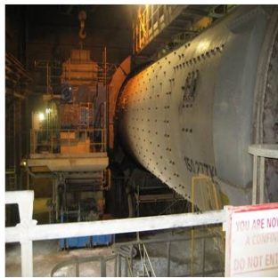
Cement mill with barring drive platform
