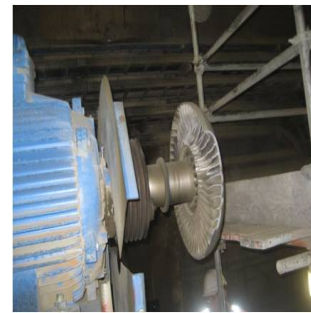
Remains of fluid coupling after failure
