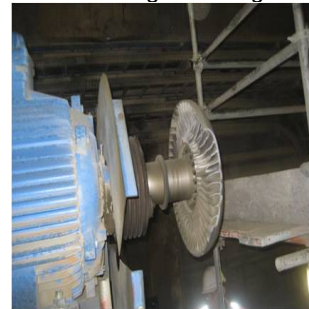
Remains of fluid coupling after failure
