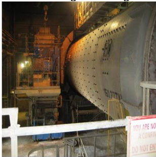
Cement mill with barring drive platform
