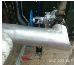
Modern system with a bleed valve which would confirm effective isolation of the pipeline
