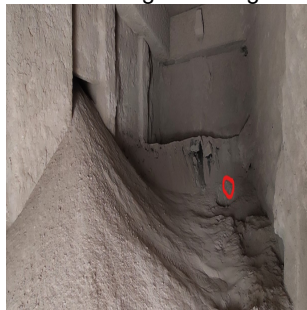
Spillage of dust
