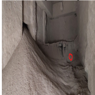
Spillage of dust
