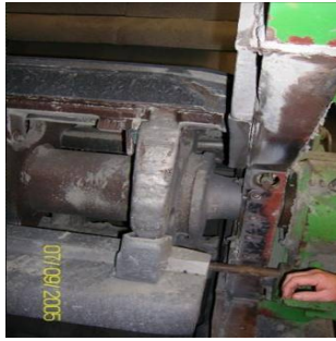
This picture shows nip point where the employees finger became trapped against the casing of the crusher and the rotor arm
