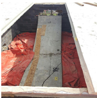
Fig. 1 - Damaged slab on ground
