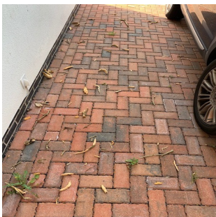
Debris in drive
