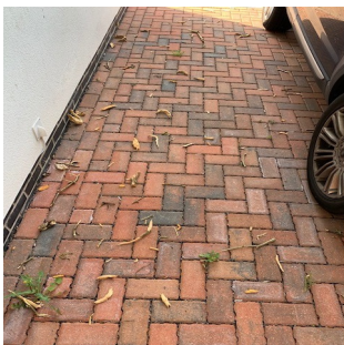
Debris in drive
