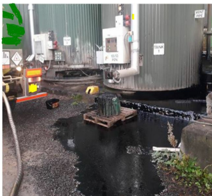
Photograph 1 - Spillage of Material
