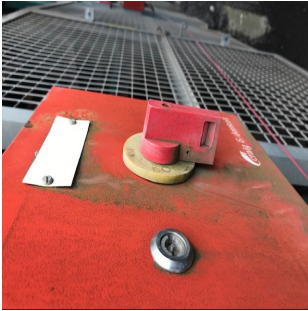
Craig and Derricott isolator
