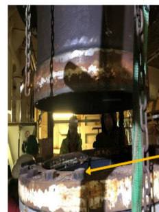
Slip flange – note bolts assumed to be securing sections
