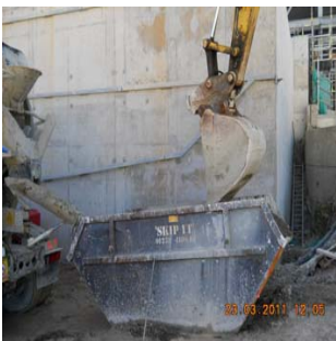
Poor Delivery Set Up
