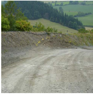
Yellow Paint Highlights Outer Wheel Path
