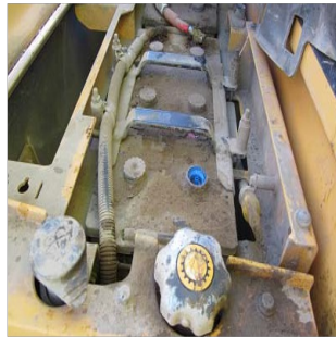
ATD Battery with Cap Missing
