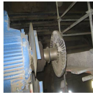
Remains of fluid coupling after failure
