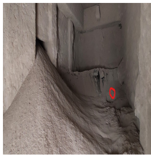
Spillage of dust
