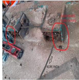
Where the wire rope was rubbing
