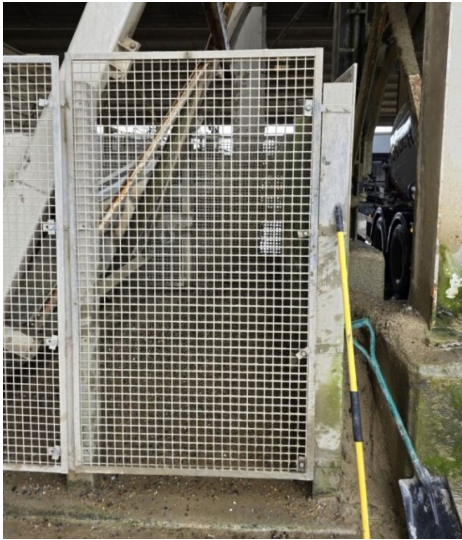
This a reverse view but showing the skip in its down position.
