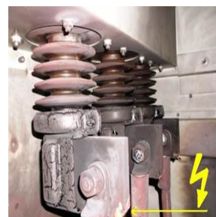
Phase to Phase Discharge
