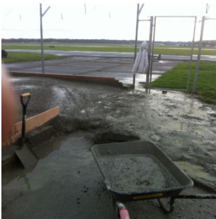
Spillage when wall collapsed
