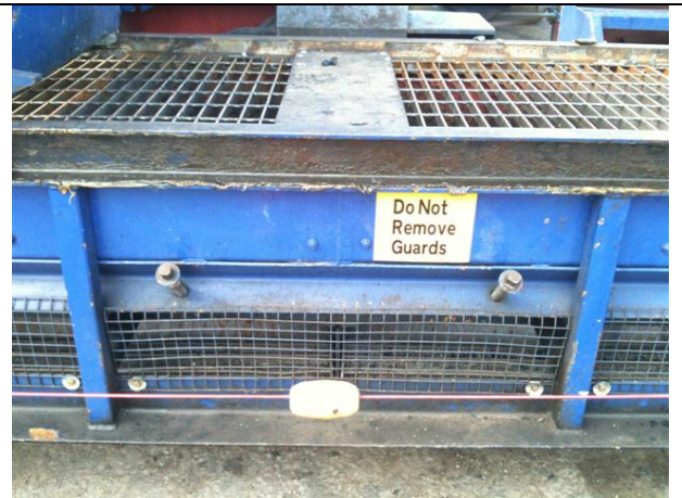
Emergency stop signs must be clearly displayed at all points where e-stops are fitted
