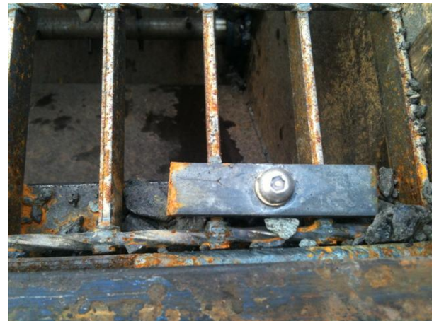
Star bolts must be used to secure the mesh in place, at 18" intervals
