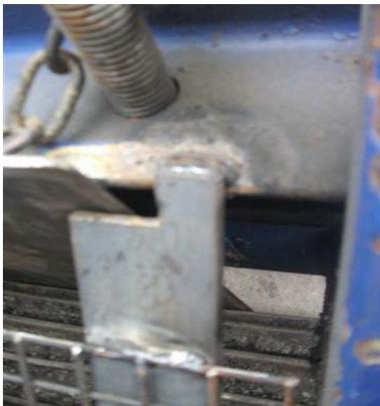
Blanking plate fully in position, resting on the back apex of the chipper trough
