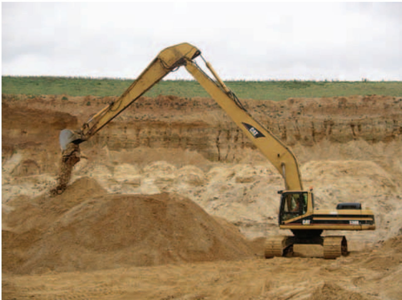
Sand and gravel quarry, Birch, Colchester, Essex. Although the excavator may move slowly, its arm can swing rapidly through a wide arc. Close access to the area where an excavator is working presents a significant hazard in an active quarry.
