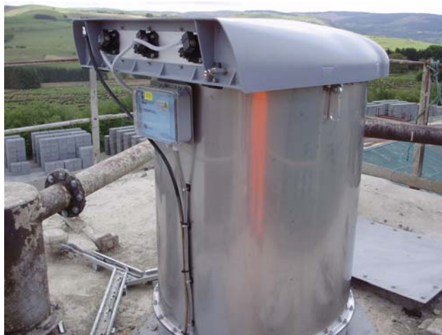
Figure 2 Filter housing on top of a silo installation
