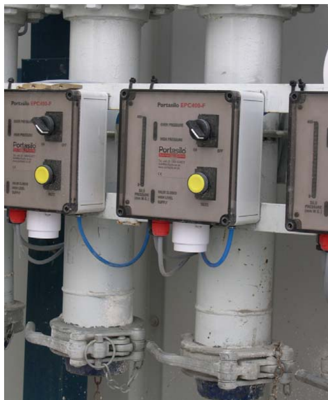
Figure 5 Bank of Automatic Shut Off Valve Controllers with Pressure Indicator and Alarm
